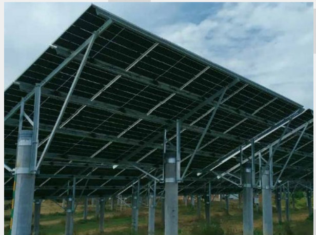
1MW Ground PV Station in Shanxi, China
