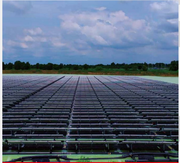
5MW Water-Floating PV Station in Bangkok, Thailand
