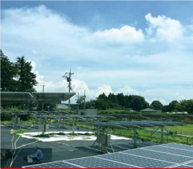
50KW PV Station in Ibaraki, Japan
