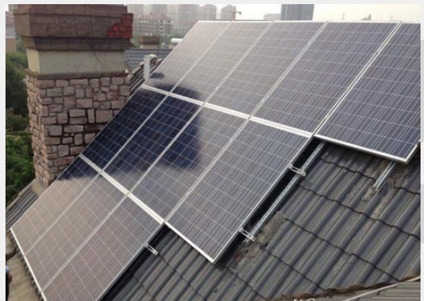
6KW Rooftop PV Station in California, USA
