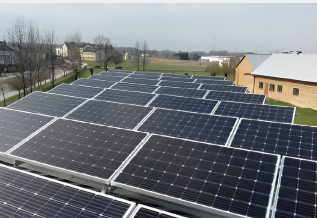
10.08kW Rooftop PV Station in Poland
