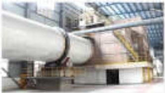
Calcining and Drying Units
