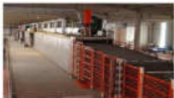
Dryer and Heat Exchanger Unit
