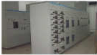
Electrical Control System
