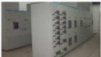
Electrical Control System
