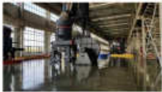
Grinding and Separation Units
