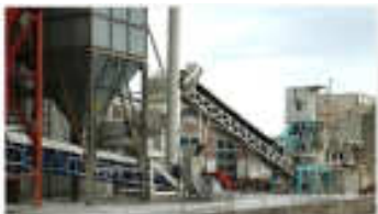
Metering and Dosing Unit
