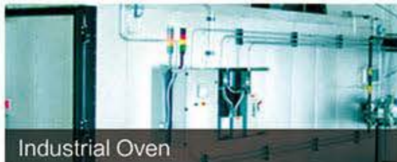
Industrial Dryer/Hot-blast Stove
