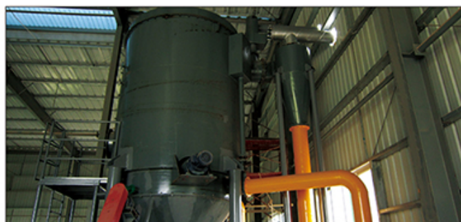
1MW UFBG POWER PLANT
