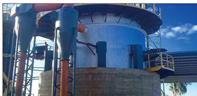
0.8MW DFBG POWER PLANT
