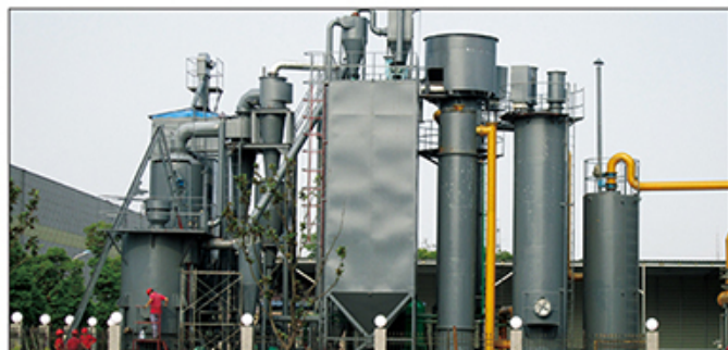
0.8MW UFBG POWER PLANT
