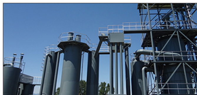
1MW TFBG POWER PLANT
