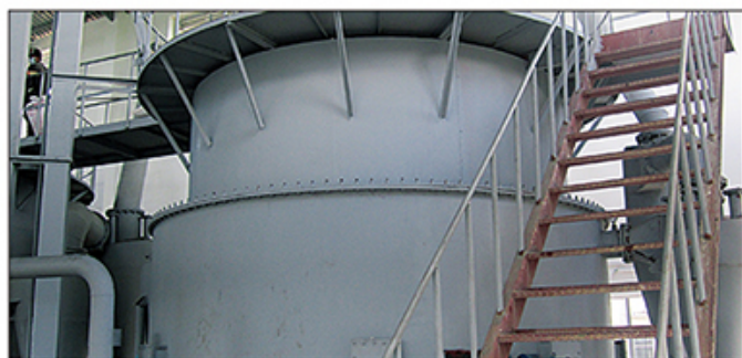
1MW DFBG POWER PLANT
