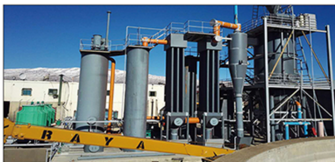
1MW UFBG POWER PLANT
