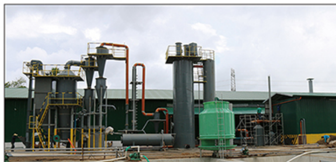
0.5MW CFBG POWER PLANT
