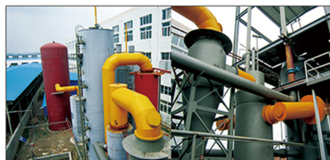
2MW TFBG POWER PLANT
