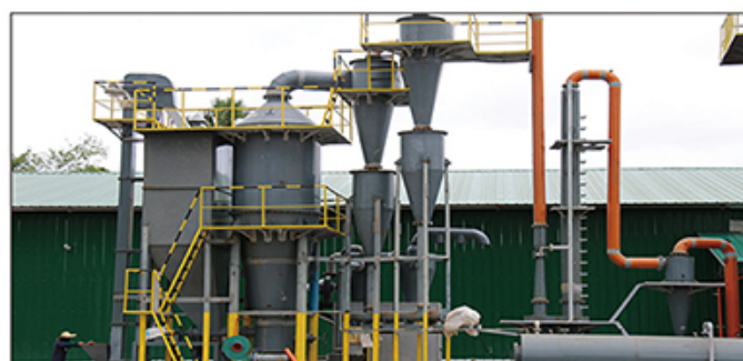
0.5MW CFBG POWER PLANT
