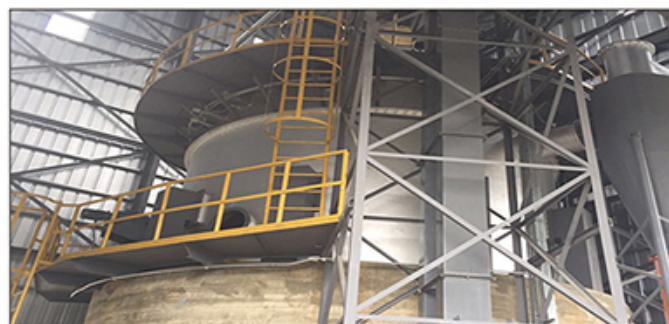
1MW DFBG POWER PLANT-2
