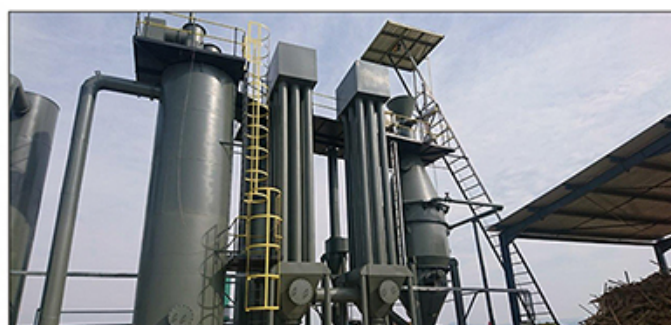
1000KW TFBG POWER PLANT
