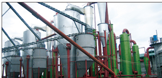
3MW CFBG POWER PLANT
