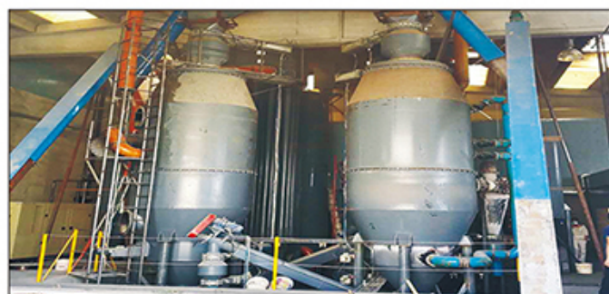
2 x 200KW TFBG POWER PLANT
