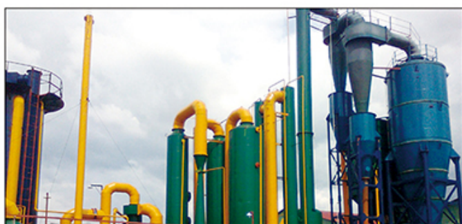
2MW CFBG POWER PLANT
