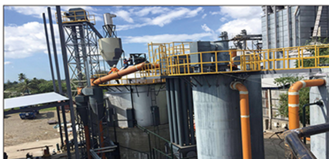
1MW DFBG POWER PLANT
