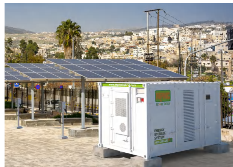
EV Charging Solar + BESS
