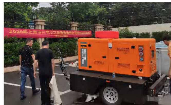
Shanghai, Perkins, Emergency
