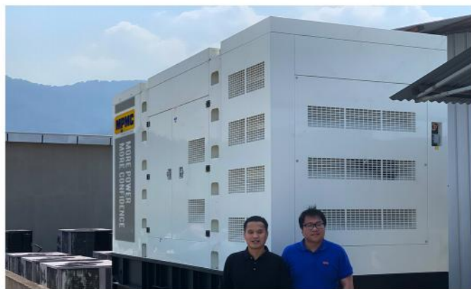
Honduras, Cummins, Standby
